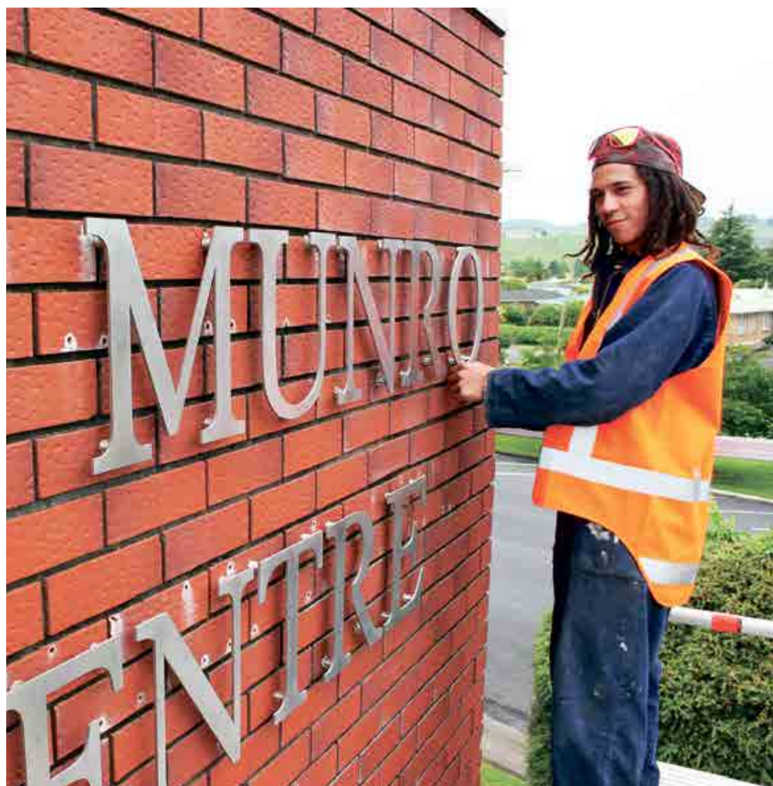
O FOR OFFICIAL: Kenedy Strachan (22) of Otorohanga's Detech Engineering puts the last letter on the new signage of the former Waitomo Cultural and Arts Centre. It now bears the name of the past mayor, Les Munro, who died in August. Other signage was completed by Signs Alone of Te Kuiti.
