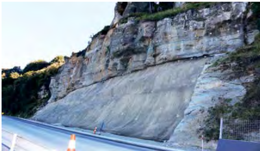
ANCHORED: After seven months, the $2.5 million New Zealand Transport Agency project to secure a section of the Mangaotaki Bluffs on SH3 is finished.
