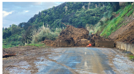
Pukerimu Road slip
