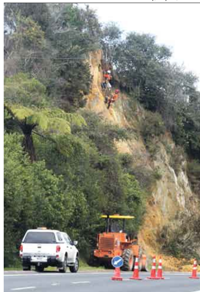
HANGING OUT: Traffic was held up for brief periods on Friday as two industrial abseilers worked up a steep cliff face beside SH3, one kilometre south of the Hangatiki intersection. Transfield Services manager Gareth Bellamy says specialist industrial abseilers were hired to chip away loose overhanging sandstone which could potentially fall onto the highway. "It's just routine SH3 maintenance as far as Transfield is concerned." The experts from Hamilton company Avalon Abseiling removed two truckloads of sandstone from the steep cutting. Traffic control was provided by Inframax staff to enable the abseilers to work safely and give trucks access to the site.
