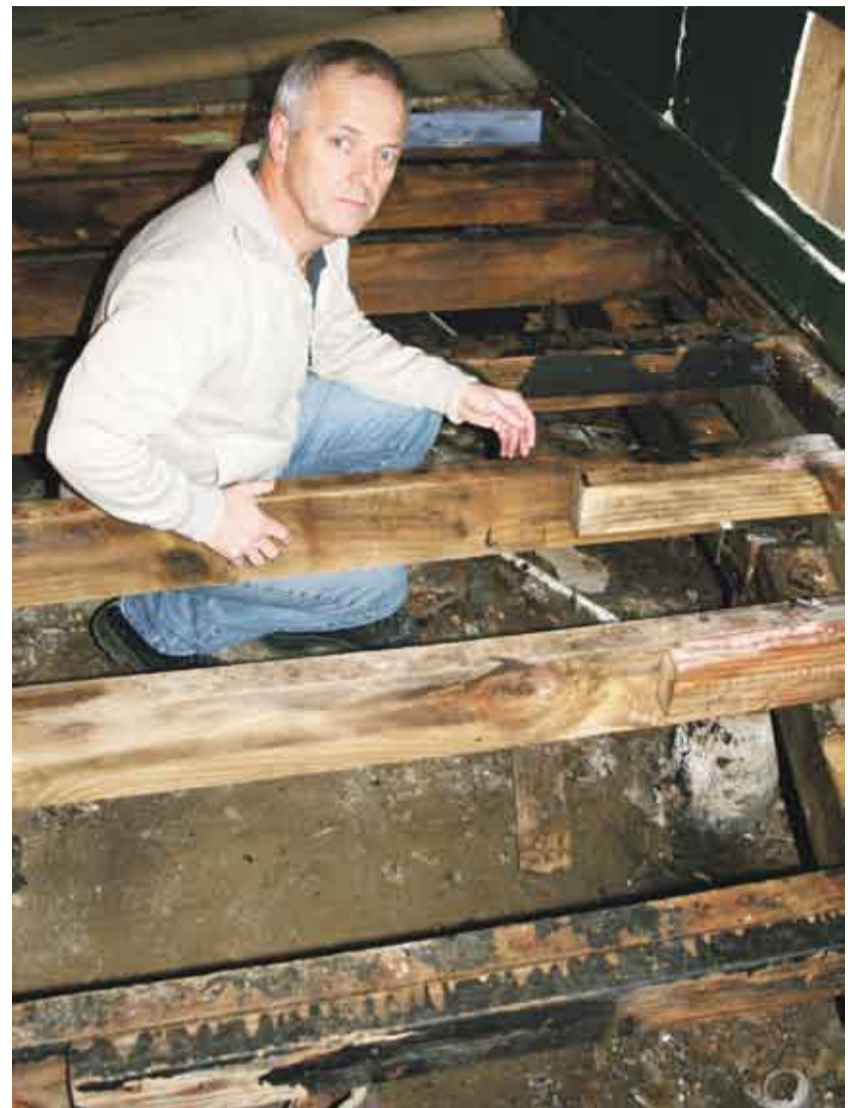
ACTING UP: Te Kuiti On-Stage theatre group president Rob Blamires inspects the damage probably caused by water running off the adjacent stadium carpark.
