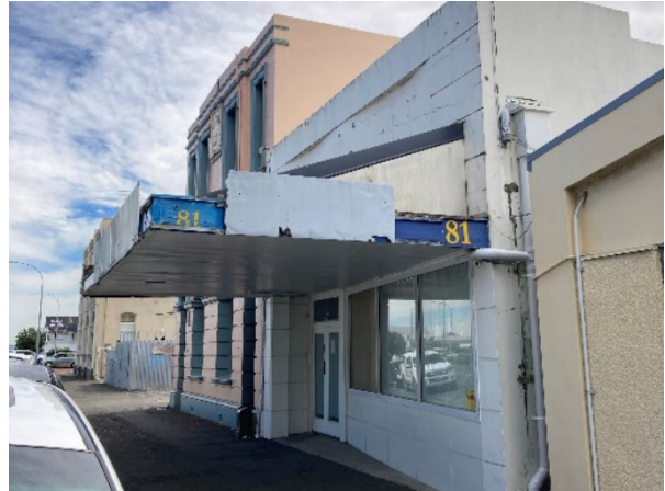
Deteriorating building. Childers Rd
