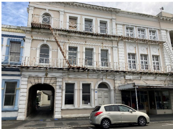
Masonic Hotel decaying façade. Lowe St
