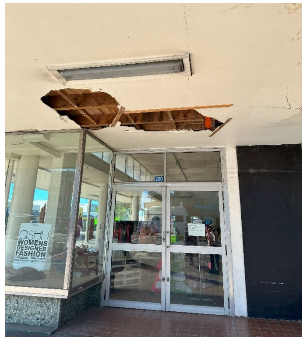
Main Street building decay. Gladstone Rd
