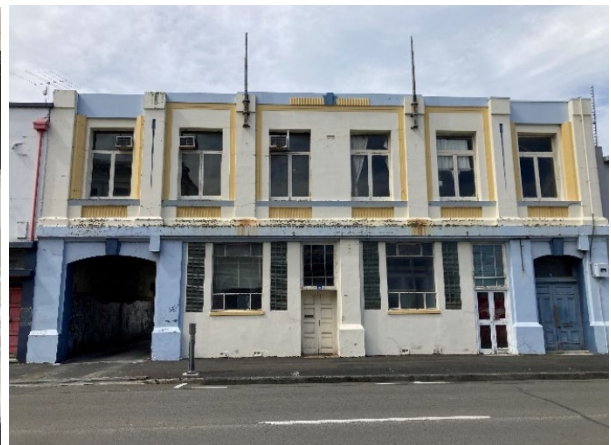
Deteriorating building. Lowe St
