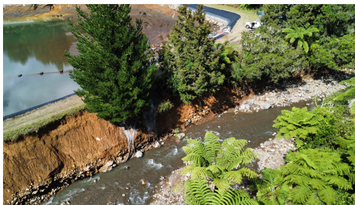
Flooding caused multiple slips in the Mangauika Stream and destroyed the water treatment plant's intake structure.
