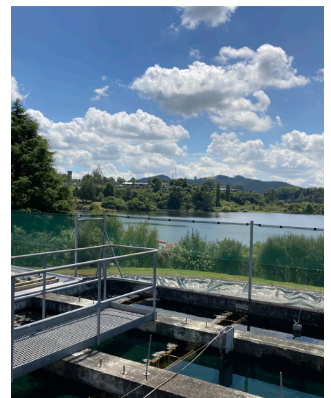
Karapiro Water Treatment Plant
