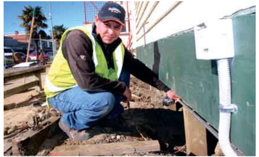
ON TRACK: DML Builders (2003) Ltd foreman Stephen Kite is overseeing the external restoration stage of Waitomo District Council's Railway Buildings Revitalisation Project.
